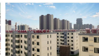
Compact solar energy project, Siji Jiayuan, Haigang Development Zone, Tangshan, Hebei Province
