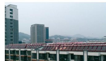
Compact solar energy project in Jingdu Garden Community, Zhangjiakou, Hebei Province
